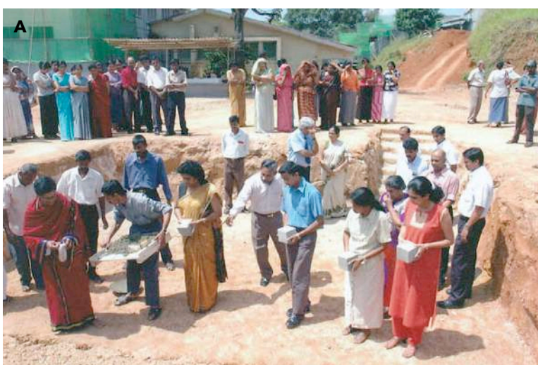
A. Laying the foundation for the new paraclinical building on February 15 th , 2006. Front - L-R Hindu Priest, unknown, unknown, Mr. Eng. Ariyaratne, Anupa Herath ( MFSU president), Miss Sujatha Ramadasa, Dr. Pushpa Idirisinghe (PGIM trainee) Dr. Deepthi Edussuriya. Behind Deepthi, Mr, Eriyagama and Mr. R.L. Ranaweera. The VC Professor Kapila Gunasekera and Neelakanthi Ratnatunga (green and white saree) standing near the steps, planning the next strategy. Far back right tope - Prof PAJ Perera and Prof Malakanthi Chandrasekera (Back view). Far back - Members of the non academic staff.
